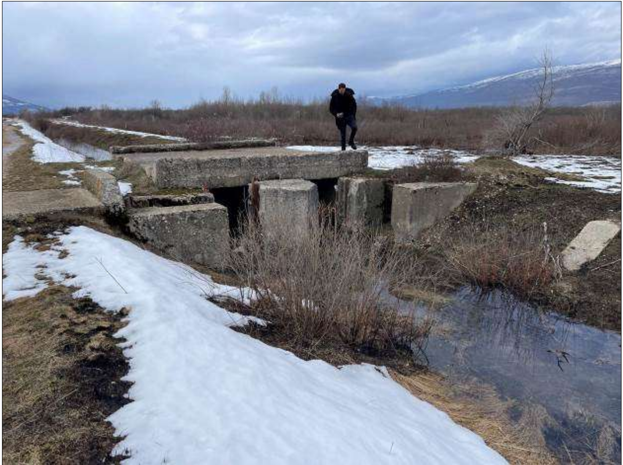
Slika 8. Segments of the drainage channel where small bridges with weirs are constructed.
