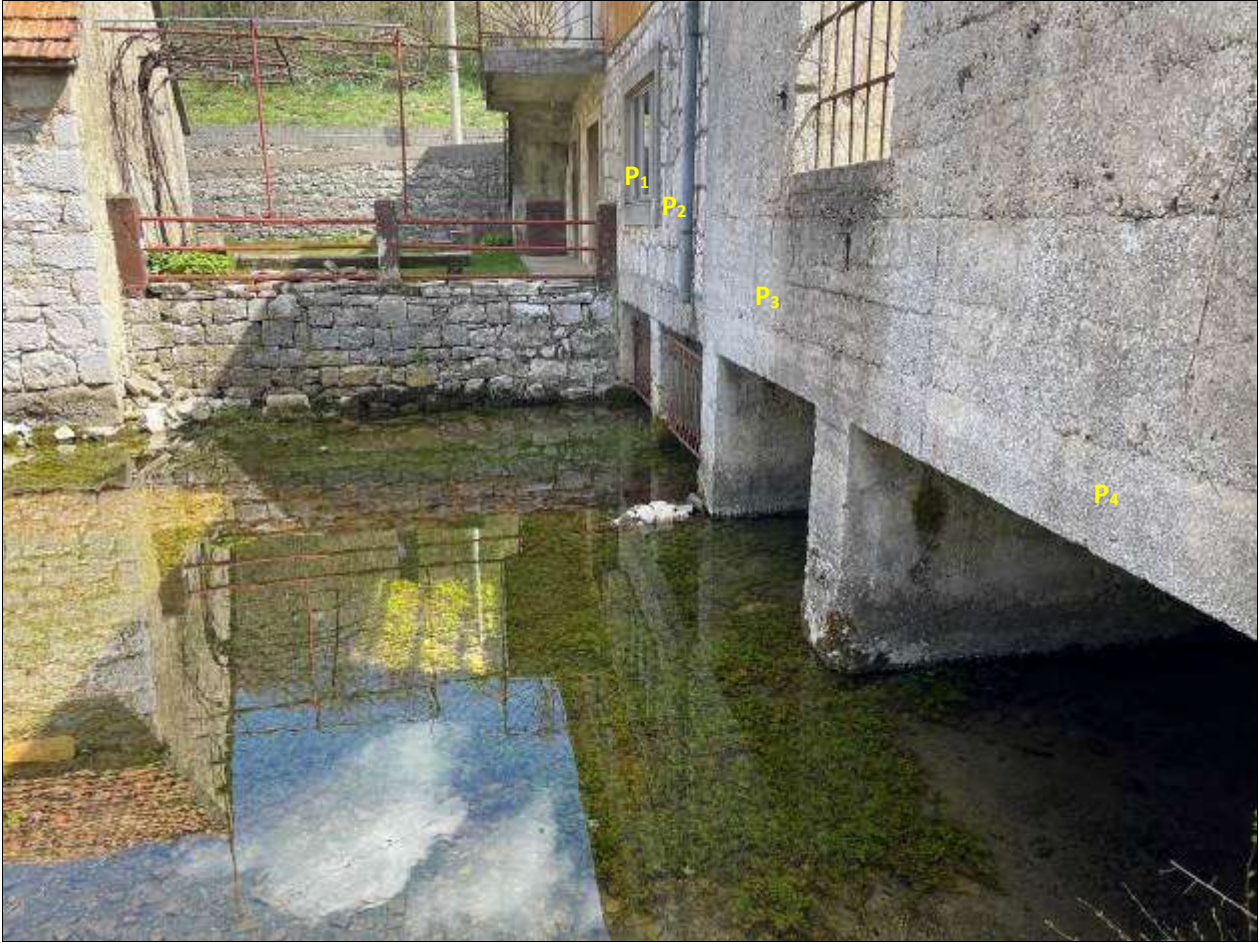
Picture 18. The front part of the space on the load-bearing walls of residential building 2 and auxiliary building 1 where the removal barriers are constructed.
