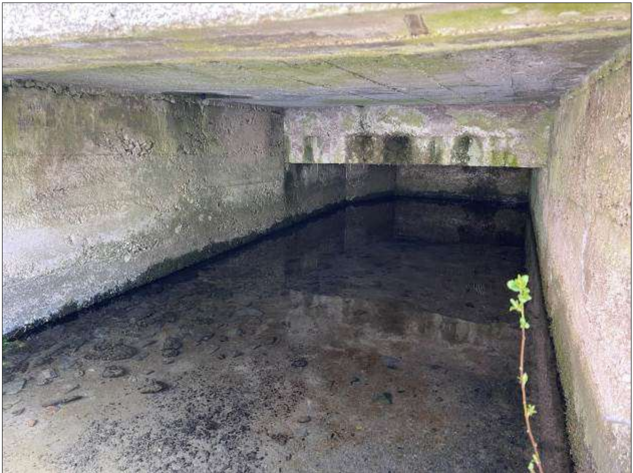
Slika 20. View of the rear part of the load-bearing wall in auxiliary building 1, where barrier no. 4 for removal is constructed.
